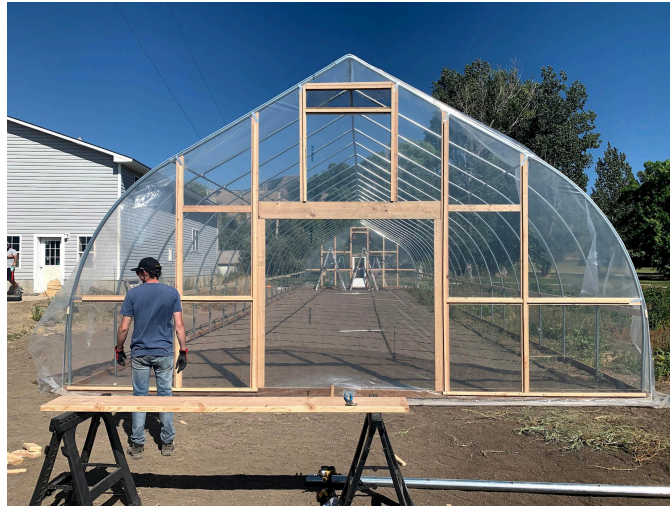
Figure 10 – High tunnel with framing finished. Note opening for a bay door and storm door.
