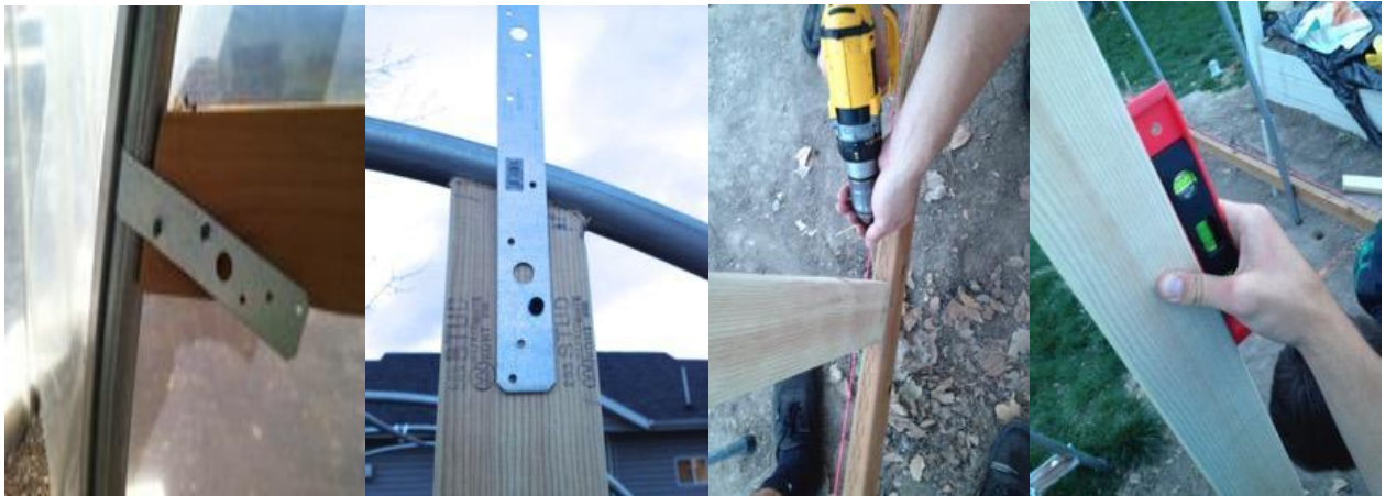
Figure 21 – Framing ends of hightunnel (Metal straps looking from the inside, on far left).
