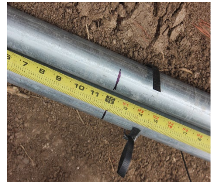
Figure 4 – 12” Marking on posts
